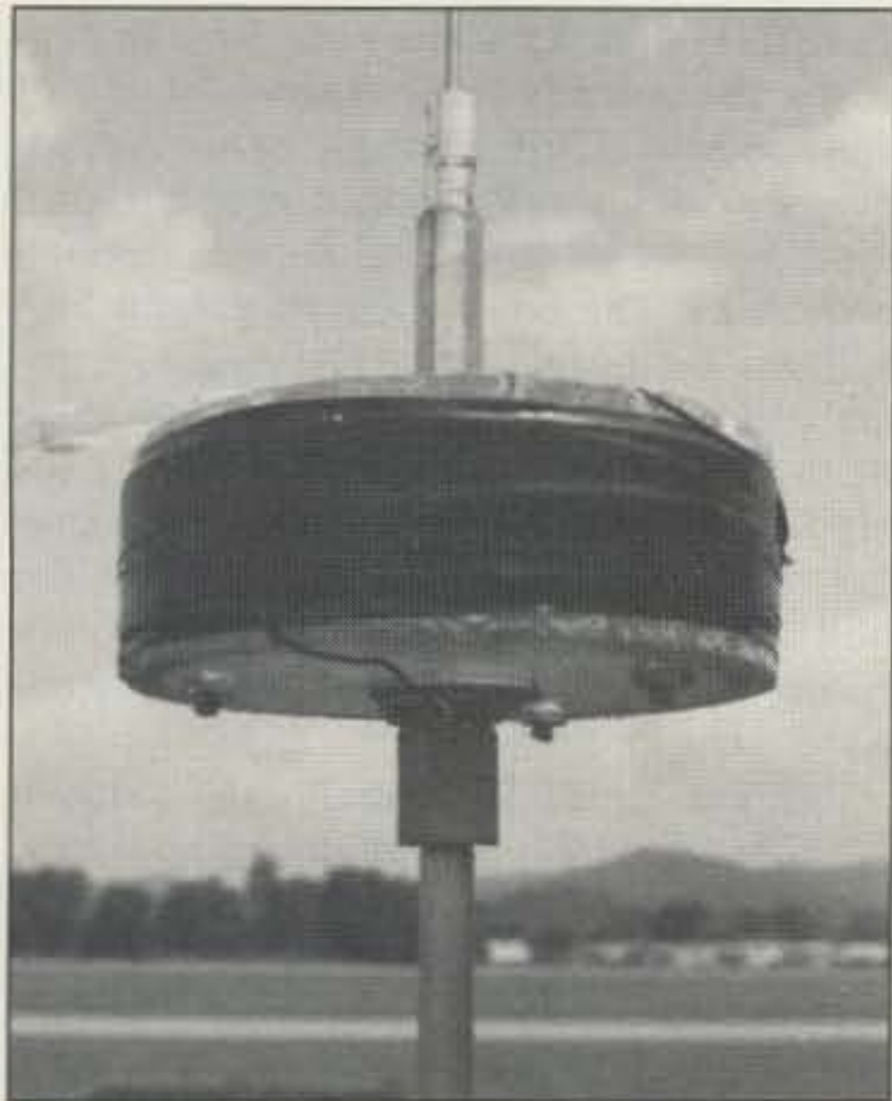
Photo B. Close-up view of the loading coil.
