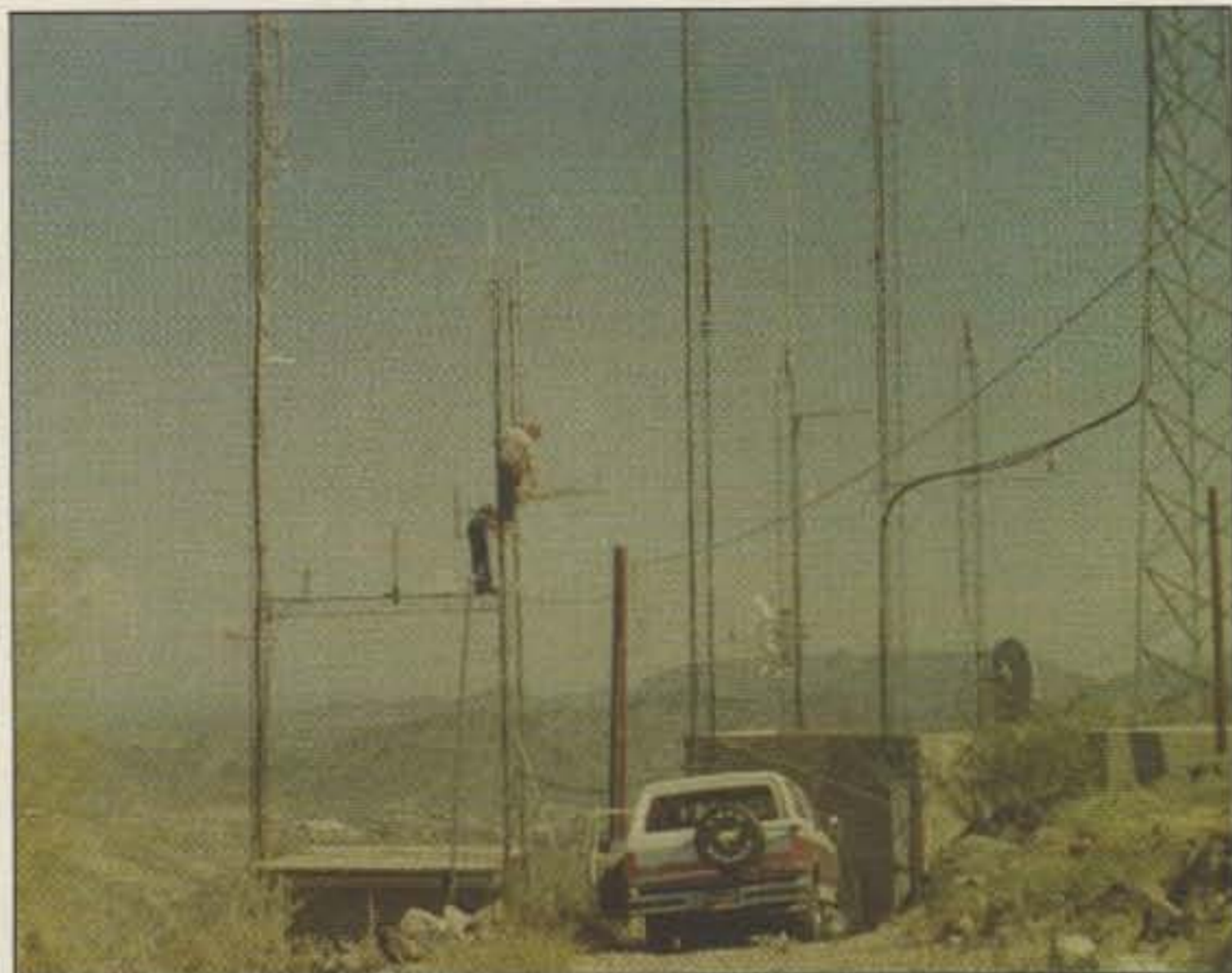
Photo D. KS8J ATV repeater site on top of Shaw Butte overlooking greater Phoenix. Roger KD7HH and Wayne N7MAO can be seen installing the new antennas.
