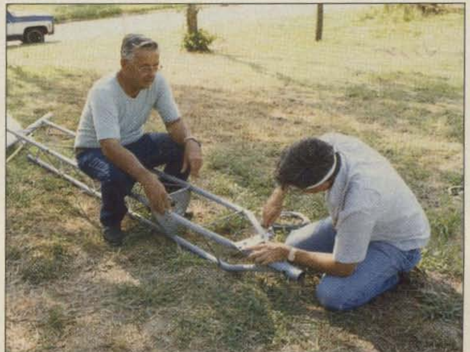
Photo B. Hazer rope wire pulley assembly installation at the top of the tower. We installed the Hazer during the tower installation.
