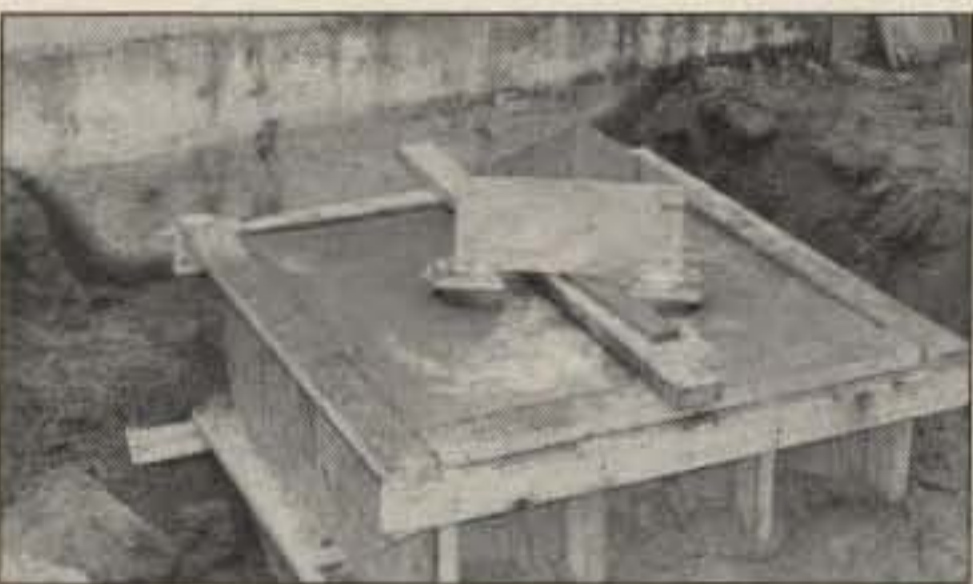
Photo B. The area around the form is partially backfilled after the concrete has been poured.
