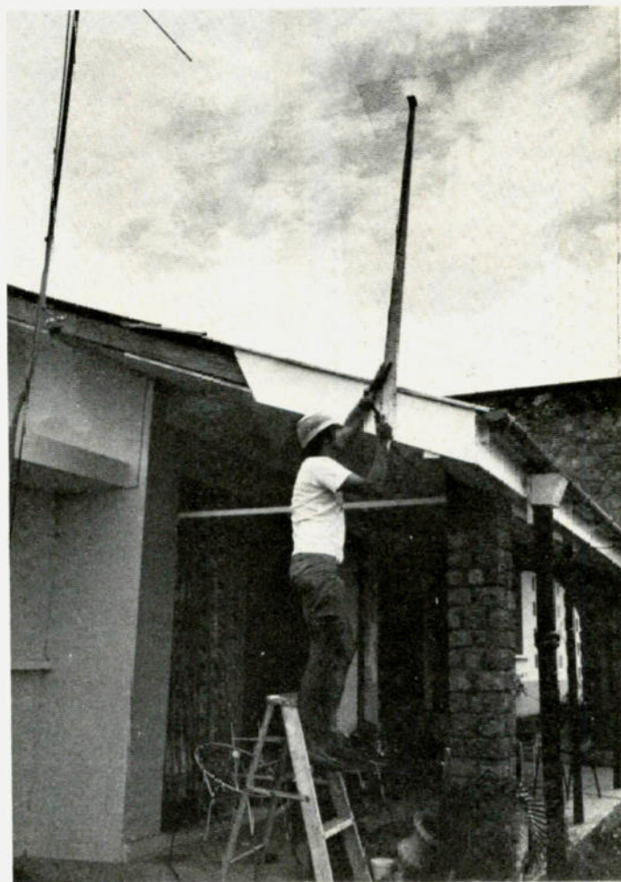
Photo M. Erection of a 2-meter quarter-wave vertical with a chicken-wire ground plane.
