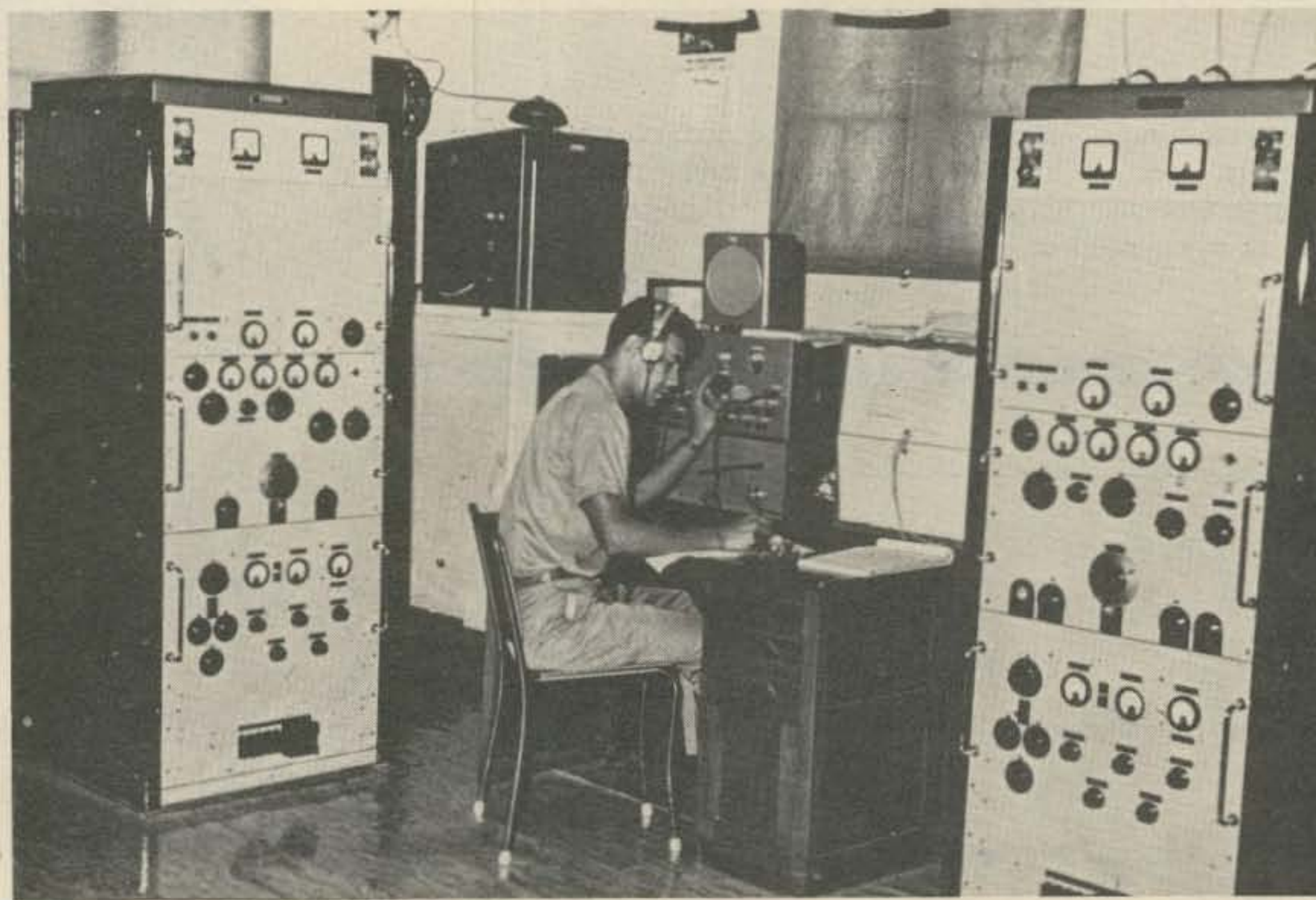
Tom Christian on duty operating Pitcairn's radio station "ZBP." The equipment is British with a power output of about five hundred Watts. Tom operates, maintains, and installed the station. Two daily overseas schedules are kept with Auckland, New Zealand. Cablegrams on an international basis are received and transmitted on an average of one hundred per month. The marine radio, also at the station, is used to contact ships at sea, some of which stop at Pitcairn. All traffic from "ZBP" is by CW mode. Tom and Betty both have a code speed of twenty-five words per minute.
