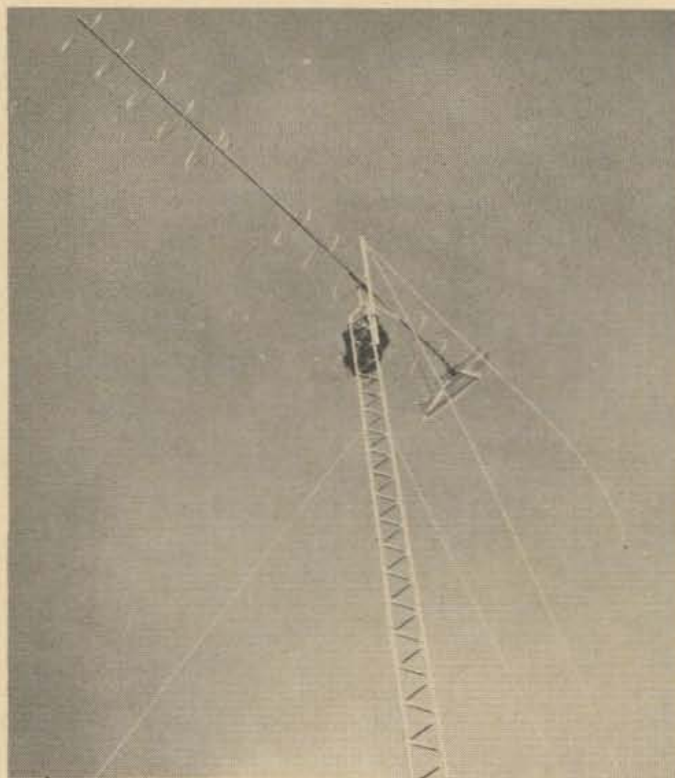
Fig. 4. The array is in position, with ropes gleaming in the sunlight. Use of a rugged gin pole is an essential.
