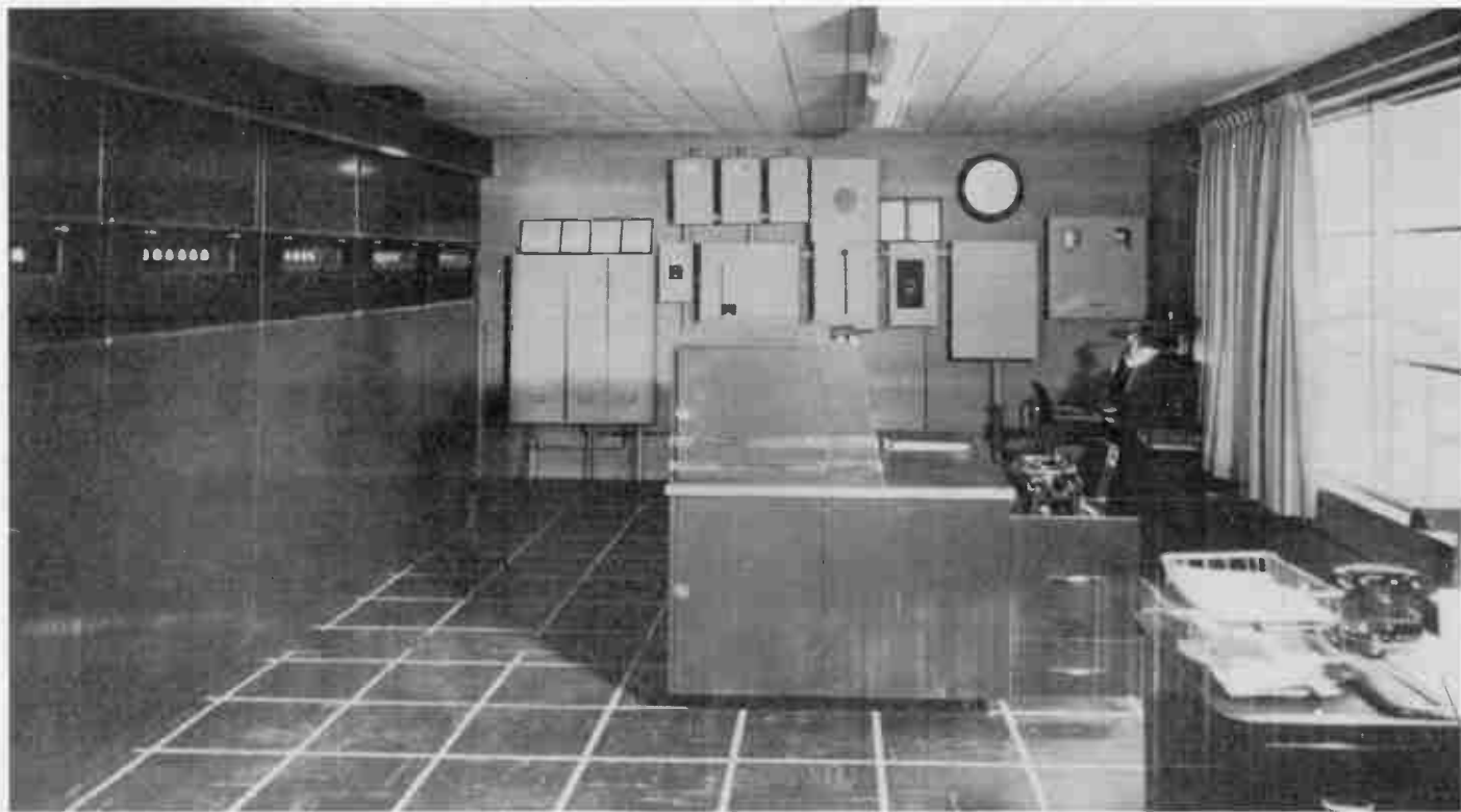
Interior of the Transmitter Building of DuMont Station WDTV at Pittsburgh.
