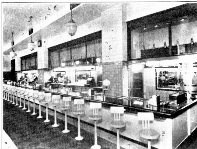
Fig. 8. Interior view of a modern air-conditioned lunch-room. Note the air delivery ducts and openings along the ceiling. Air-conditioned eating places are much more popular and generally do a much greater business than those that are not so equipped. Courtesy York Ice Machine Corporation.
