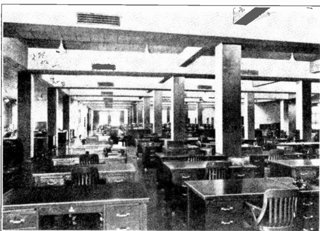
Fig. 148. Photo of the inside of a modern air-conditioned general office. Note the duct outlets along the ceiling beams. Much better efficiency and health can be maintained in such air-conditioned offices. Courtesy Jewell Tea Co.
