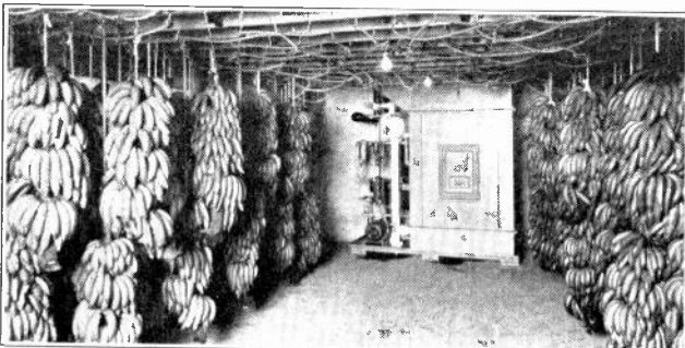
Fig. 5. Interior view of a refrigerated room used for cooling and storing fruits. Note the refrigeration unit in the background. Courtesy York Ice Machine Corporation.
