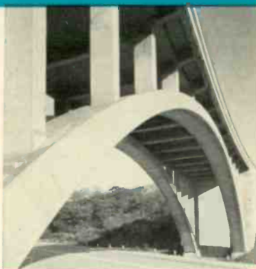
This reinforced concrete arch bridge (right) spans the Penn-Lincoln Parkway in Pittsburgh, Pa. The bridge is 251 feet long and rises to 40 feet above the roadway.
