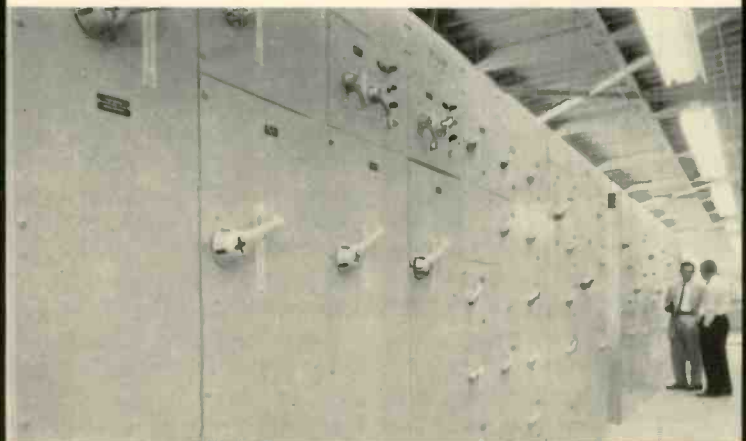
Control centers for auxiliary 440-volt motors.
