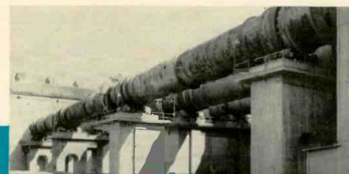
These huge rotary kilns are the heart of the cement processing plant. Once fired, they run continuously 24 hours a day, 7 days a week. All processes are geared to keep the kilns in operation.
