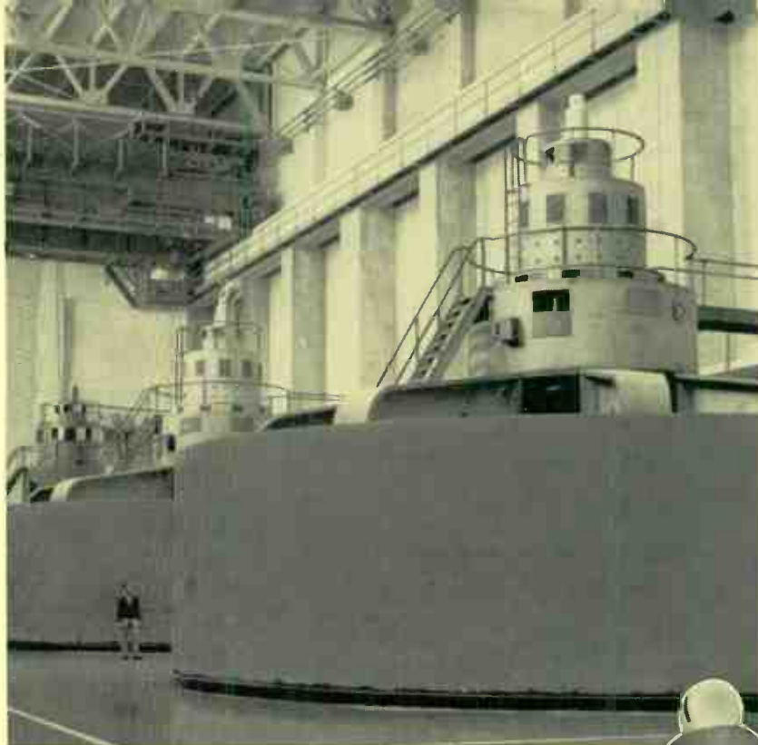
The main waterwheel generators at Grand Coulee, each rated at 108 000 kw, are the largest electrically in the world.
