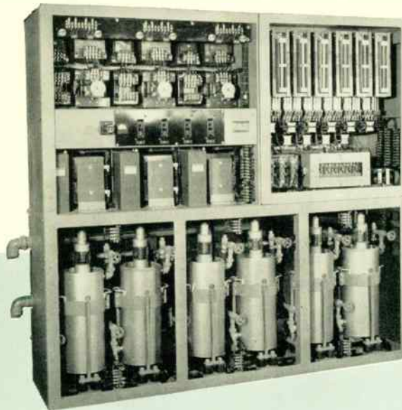
Fig. 4—Each ignitron cubicle houses six tubes and associated apparatus. Tube-firing controls are at the top left; anode breakers, upper right.
