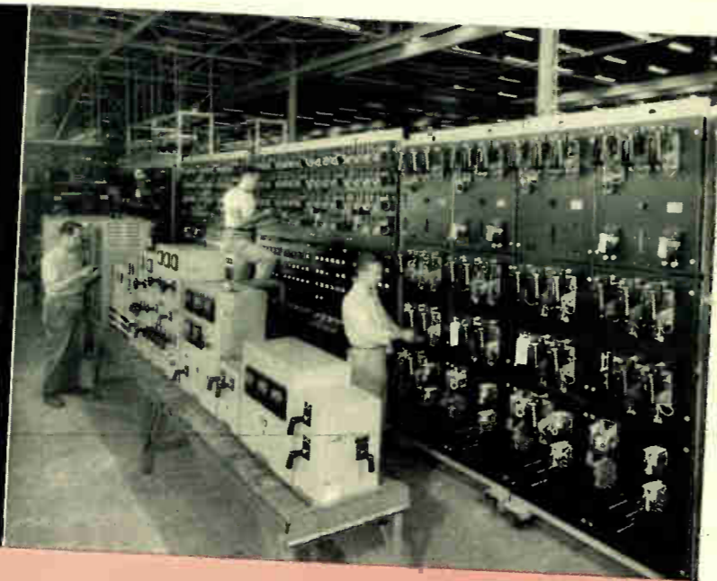
One section of the control equipment of a new tandem cold mill that is part of France's expanded steel-making facilities.
