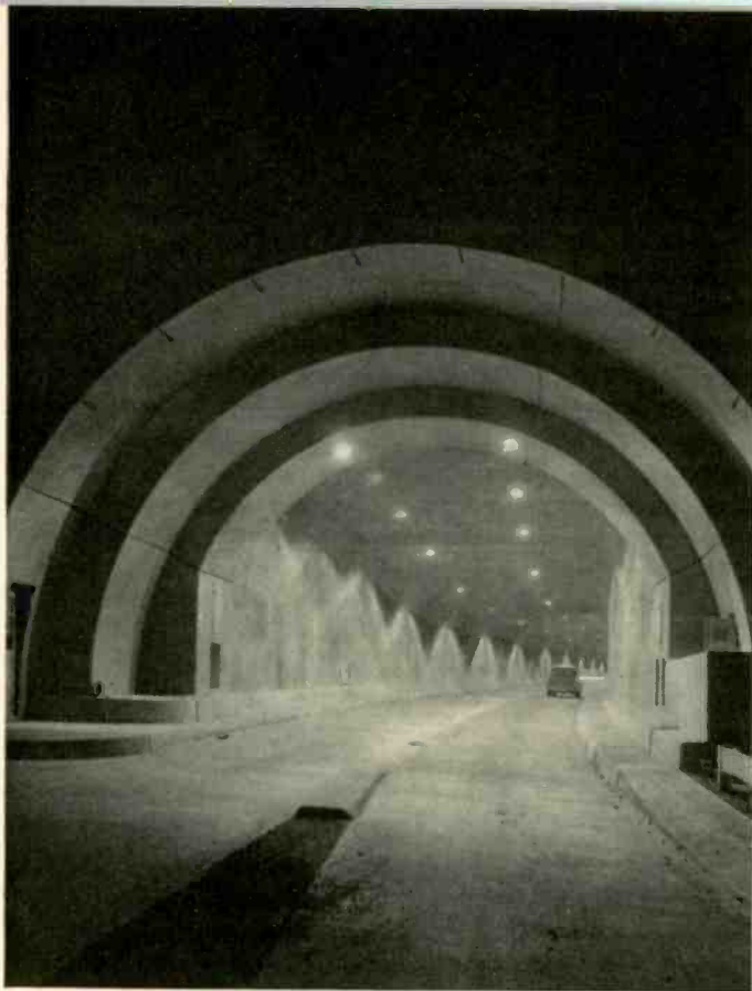
Fig. 2—Six years of service with quartz mercury lamps in the Pennsylvania Turnpike Tunnels reveal a high degree of economy and dependability. The spacing of the lamps achieves good illumination of the roadway with the smallest number of units.
