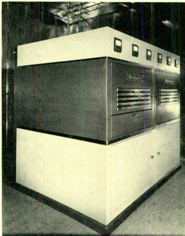
This cabinet houses both the high-frequency oscillator and its rectifier. The rating is 200 kw at 1.7 megacycles.
