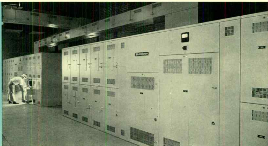
Auxiliaries at the Windsor station of the West Penn Power Company are controlled by this new 460-volt metal-enclosed switch-gear. Each of its three sections has a 4000-ampere main breaker, a 3000-ampere tie breaker, and twenty 1200-ampere feeder breakers.
