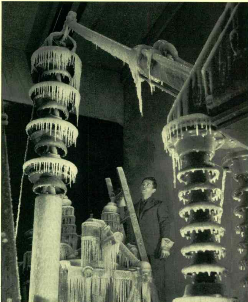
A compressed-air circuit breaker being tested at -10 deg. F.
