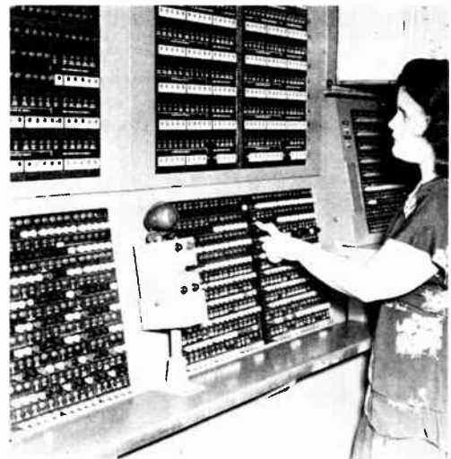
Figure 69. Connection indicator board
