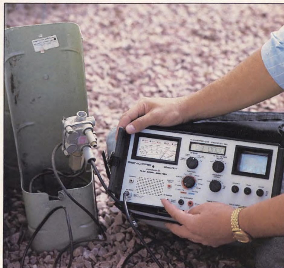
Fig. 5: Since the FS74 monitor is powered from batteries, you can check for interference at any point in the distribution system.
