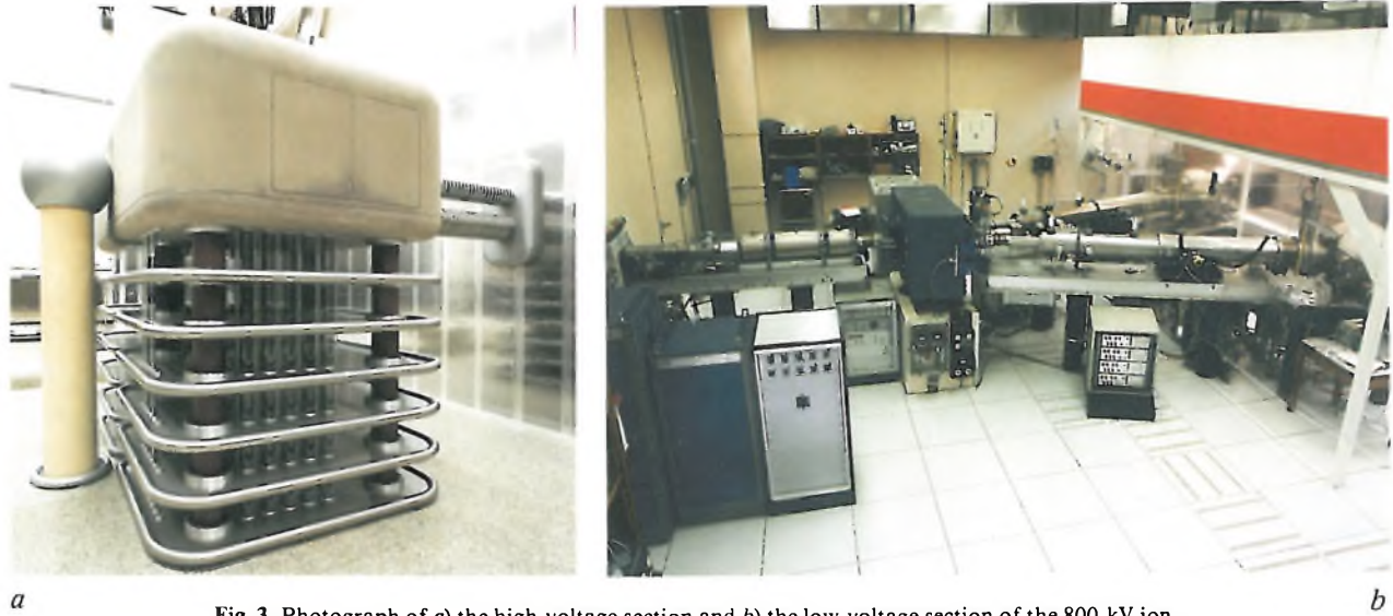
Fig. 3. Photograph of a) the high-voltage section and b) the low-voltage section of the 800-kV ion-implantation machine.
