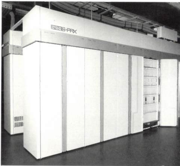
Fig. 17. Two suites of racks from the extremely modern digital processor-controlled 5ESS-PRX telephone-switching system. Here 'electronification' is complete: both the switching network and the control system consist of electronic rather than electromechanical components. (5ESS is a trademark of AT&T Technologies Inc.)
