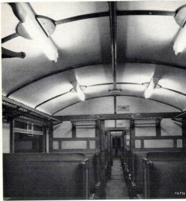
Fig. 7. Experimental installation in a carriage of the Netherlands Railways. It consists of 20 fluorescent lamps each of 20 W. Each of the lamp fittings contains a transistor converter. The supply voltage is 24 V, the frequency approx. 7 kc/s and the efficiency approx. 62%.
