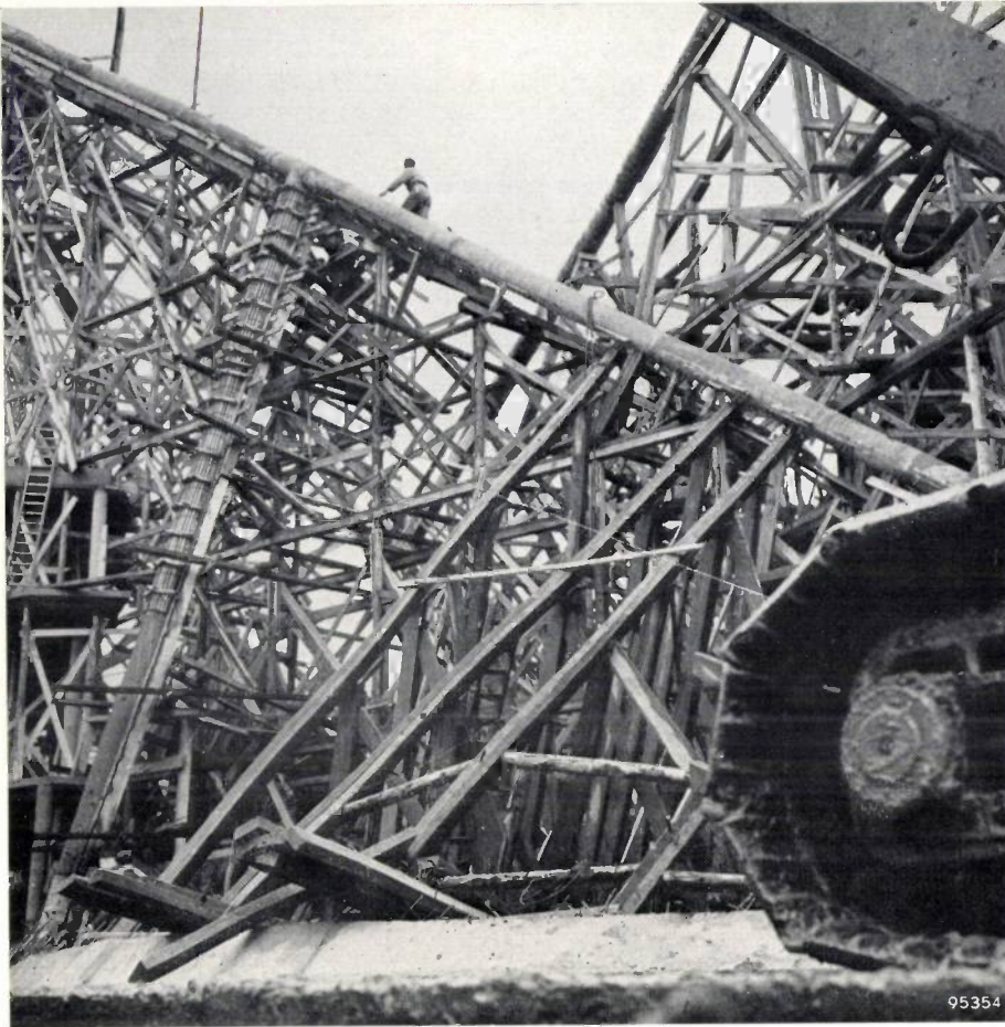
Fig. 4. The 40 cm thick cylindrical ribs were cast in situ in "shuttering" erected on scaffolding.
