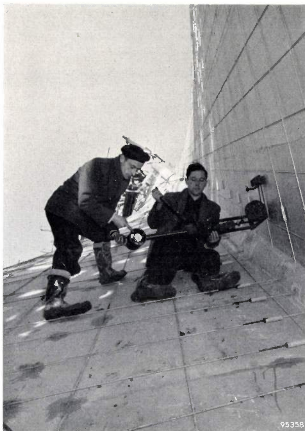
Fig. 11. Tensioning a prestressing wire with the "Strabed" jack. The tensioning force is read on a dynamometer.
