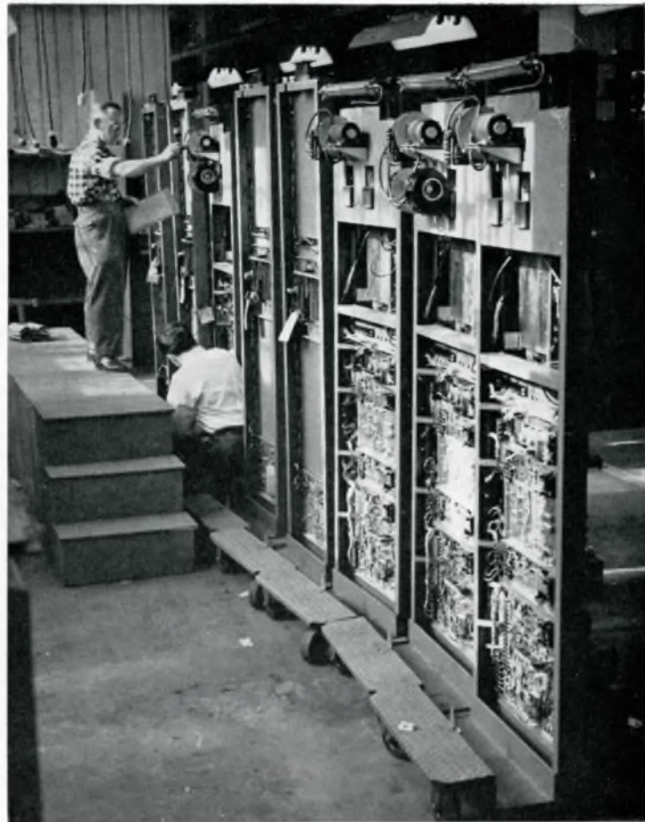
CONTINUITY TESTS are performed on a row of microwave units in the final assembly stage.
