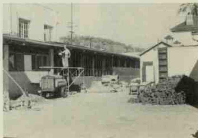
New wall being built to enlarge the room to be used by the Service department shop.
