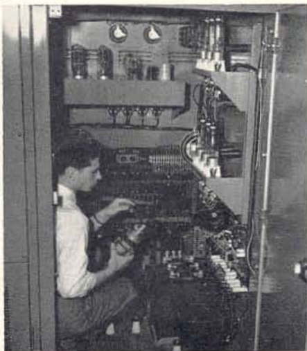
Shell Weyland, WENE Chief Engineer, readies a power amplifier tube for final installation in his Gates BC-5B Transmitter. This well illustrates the walk-in construction where any part of the new Gates 'Five' can be reached in seconds.
