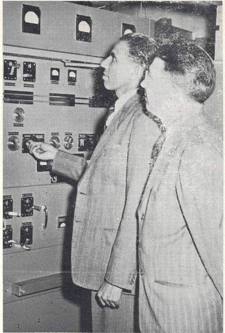
Basheer Ahmad, Deputy Director of Engineering for Radio Pakistan, inspects one of the large 10-kilowatt short-wave broadcast transmitters manufactured by Gates Radio Company which his government has purchased. Looking on is Francis Wentura, our Chief Engineer.
