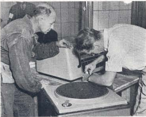
Arthur Betts, chief engineer supervises installation of Gates equipment at new station in Clearwater, Florida, WCLE.
