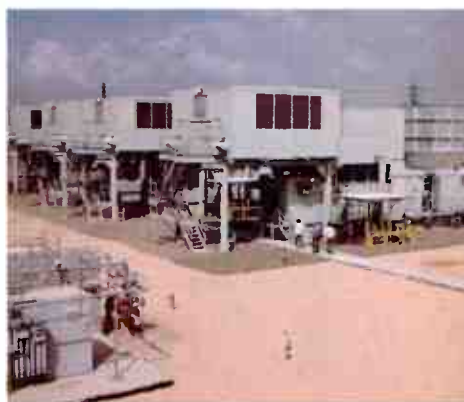
GE helps Egypt renovate its economic infrastructure. At Helwan, south of Cairo, five GE MS5001 gas turbine package power plants feed electricity into the Egyptian Electric Authority's grid.
