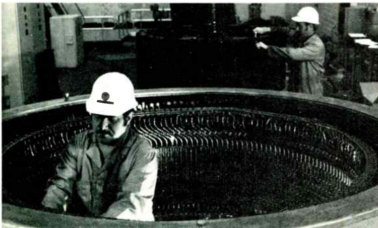
At Clinton, Mass., Service Shop’s Peter Buonauro (foreground) performs repair work inside generator stator of hydro-turbine, while Mike Tatti tightens connections on generator rotor.
