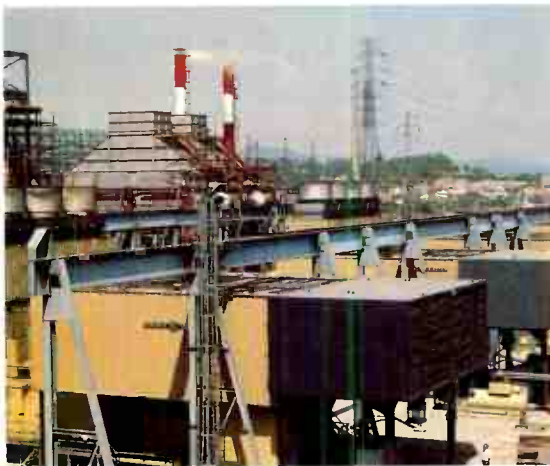
In Kunsan, GE STAG® plant
