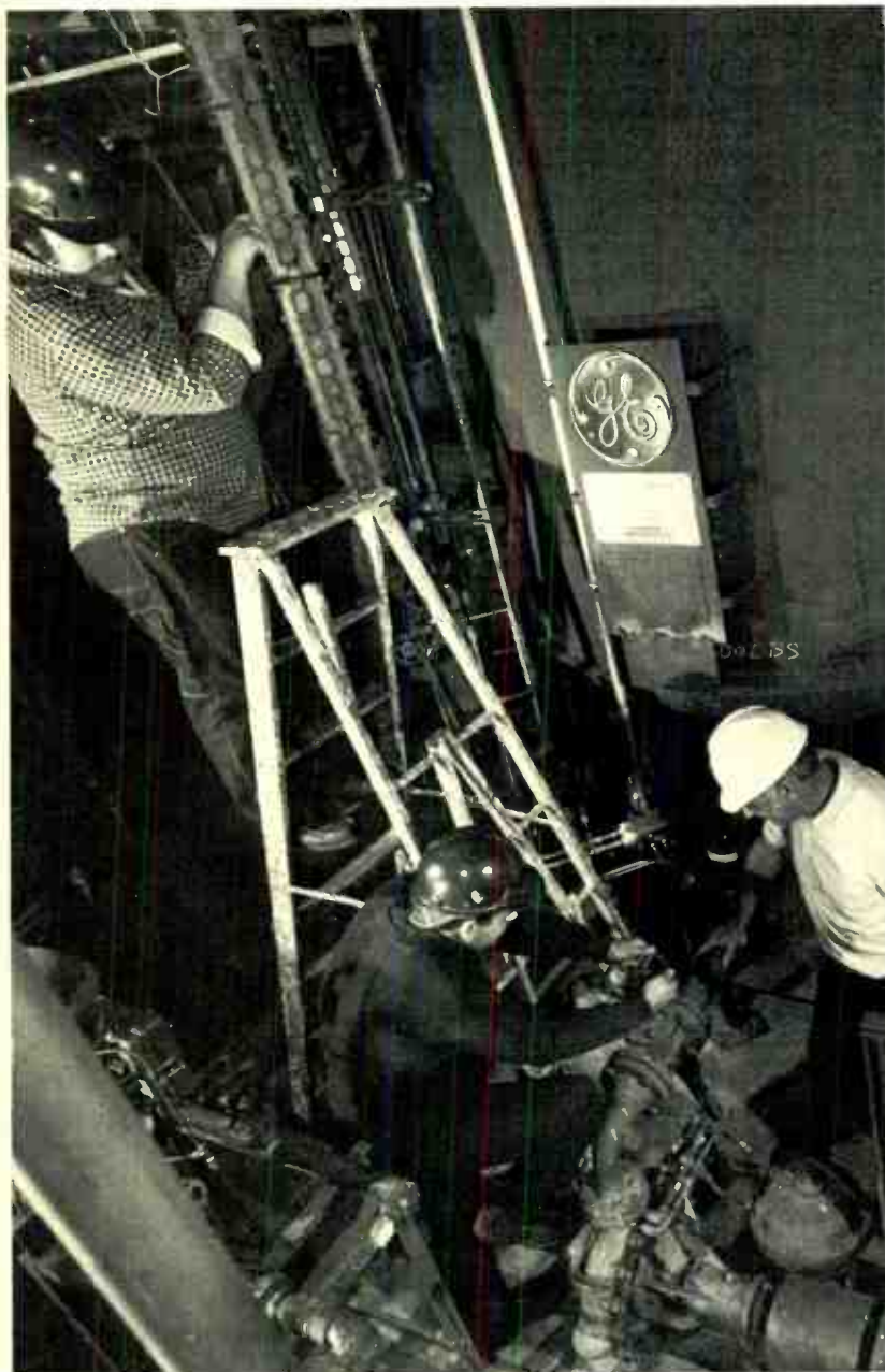
Electric production of process steam is an area of potential growth. Electrode boilers developed by Industrial Heating provide pollution-free, reliable steam production for industrial and utility applications. Shown: boiler at Brunot Island STAG plant of Duquesne Light Company.
