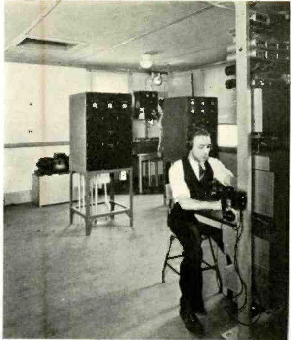
INTERIOR VIEW OF THE GREEN HARBOR STATION, MARSHFIELD, MASS., THE SENDING AND RECEIVING STATION IN THE NEW ENGLAND MARINE RADIOTELEPHONE SYSTEM.
