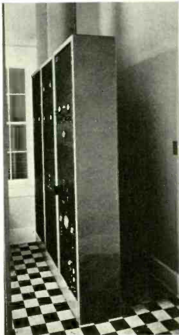
VIEW OF THE TRANSMITTER MOUNTED IN ENCLOSED-TYPE RELAY RACKS. NOTE METAL FLUES WHICH CARRY HEAT FROM THE TUBES TO THE ATTIC.
