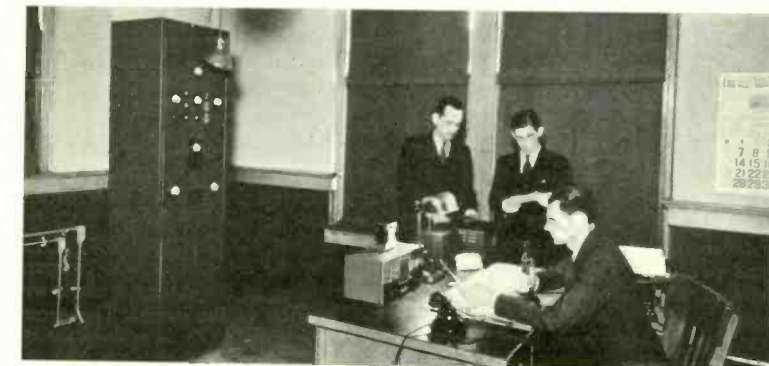
A VIEW OF THE 16-A TRANSMITTER. SEATED AT THE CONTROL DESK IS CHIEF ENGINEER McCONNELL. AT THE LEFT IS OPERATOR MORRIS WITH OPERATOR MOUTOUX AT THE RIGHT.
