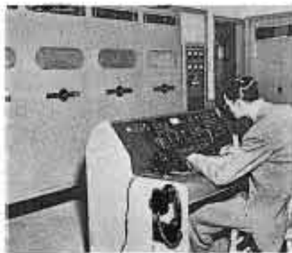
Transmitting room of WVNJ, Livingston, New Jersey, which recently went on the air. Transmitter is a 5-kw job and feeds into a five-element in-line system consisting of four towers 300' high, with the central tower 483' to the top. (Courtesy Federal Telephone and Radio Corp.)
