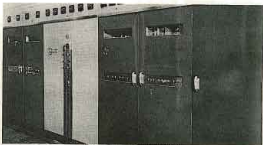
The 50-kw FM transmitter at WBRC-FM.
