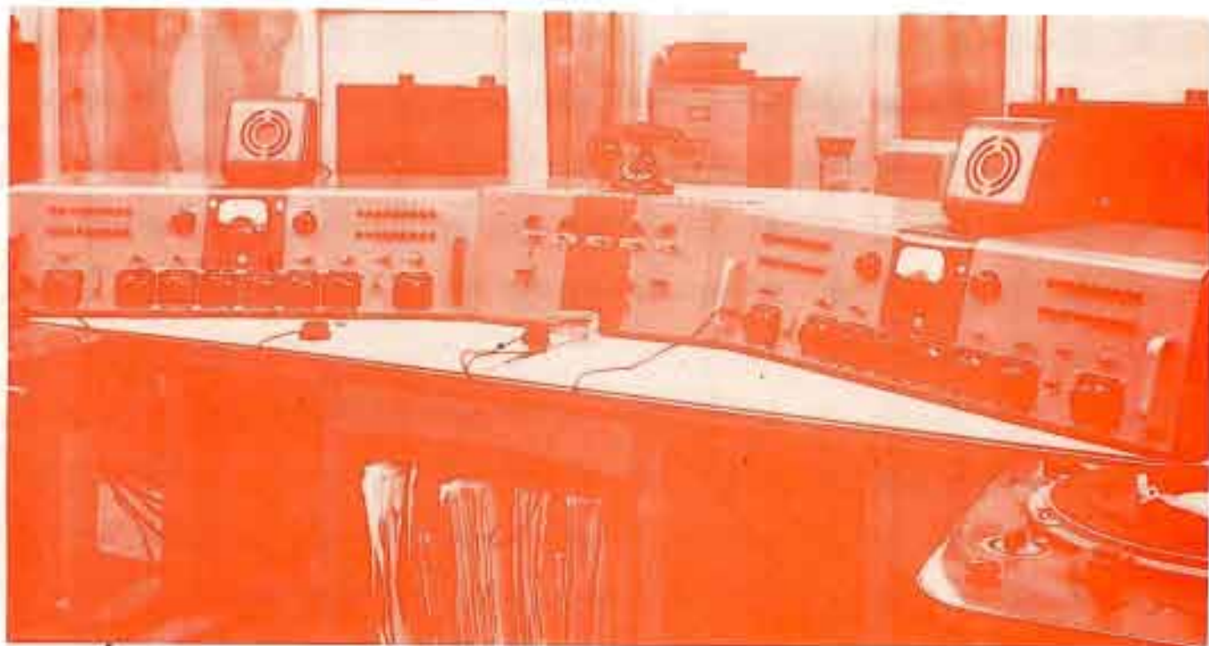
View of the completed console installation. It will be noted that a third unit appears in the middle between the two consoles. This position facilitates control by either operator. A switching system is provided so that either operator can feed either the AM or FM, or both lines by the simple throwing of a switch. The unit does not employ relays and includes a signal system in both consoles which notifies the operator which of the lines he is feeding at the moment.
