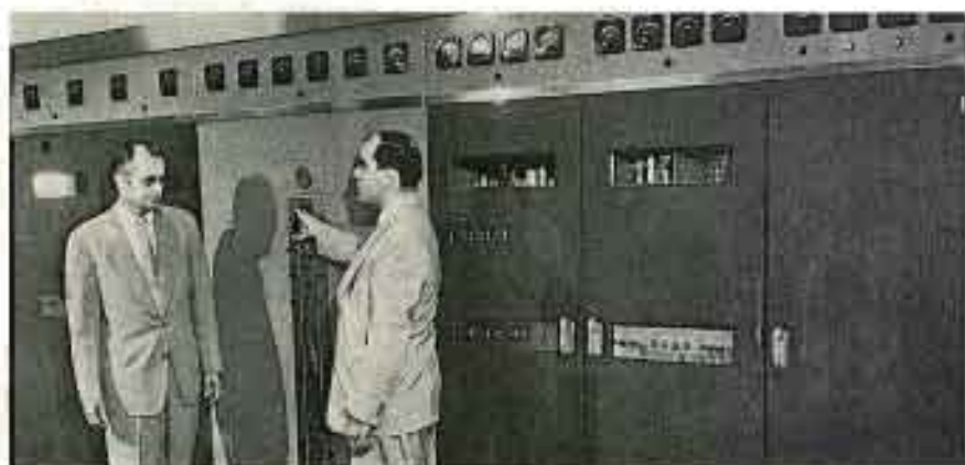
At the controls of WTMJ-FM (left to right): Phillip B. Lasser, chief engineer of WTMJ-FM and WTMJ-TV facilities and W. B. Fletcher, RCA Service Corp. engineer.
