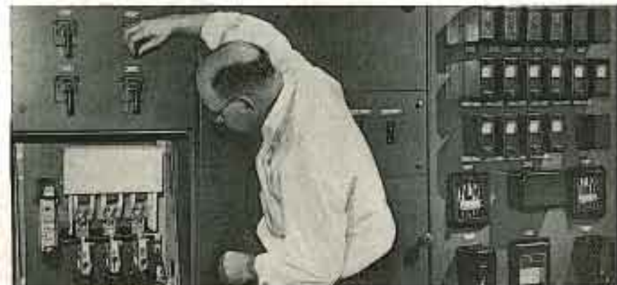
The power control and circuit breaker panel of the FM transmitter. Unit is adjacent to the 50-kw amplifier units.
