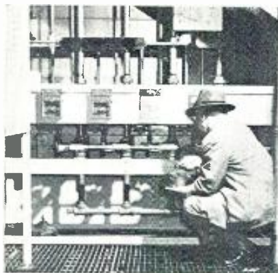
Remote control fire-fighting station located near the cylinder source. From this point additional banks of cylinders can be released manually to combat fire that might persist in upper levels after initial automatic discharge.
