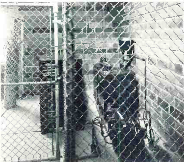
High voltage power cage. In the right foreground is a dry type plate transformer with modulation transformer and choke located adjacent. Power cage is enclosed, interlocked, grounded, and bonded for safety reasons.
