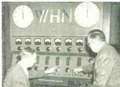
Center section of the master audio control setup being built for WHN. Equipment with six studio-control consoles and twelve audio racks will be installed in the new WHN studios at 711 Fifth Avenue, New York City. At the controls are H. J. Lavery (left) and J. F. Palmquist of the RCA broadcast audio section.
