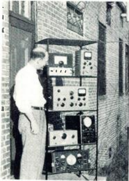
Chief transmitter operator, Joe Davenport, with a rack of test instruments. Top to bottom, left to right: Composite signal generator, vtvm, distortion meter, audio oscillator, 'scope and communications-type receiver.
