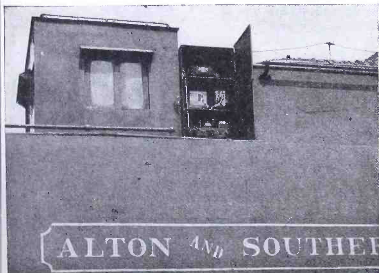
Figure 6. Railroad radio equipment in a steel cabinet on the tender. This location is better than in the cab, since the vibration is less.
