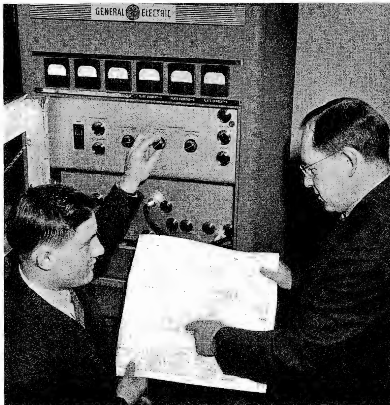
Lloyd Krause (left) discussing the engineering details of ST relay equipment recently installed by W47A, with D. S. Hoag, chief engineer of the station.
