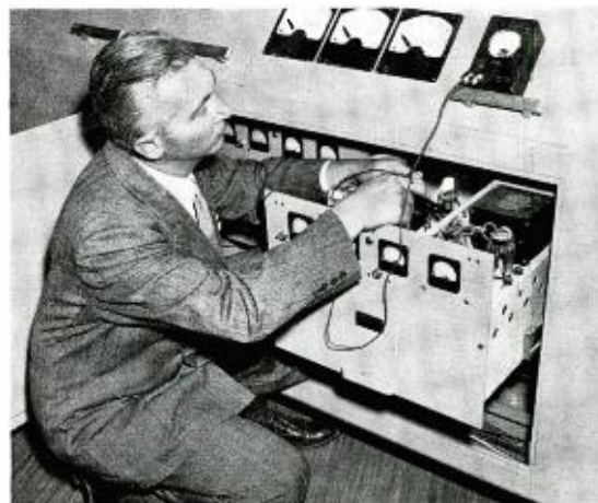
James L. Middlebrooks, engineer in charge of building the transmitter, testing one of the amplifiers, built on removable trays. These trays can be completely removed for repair while a duplicate next to it is used.
