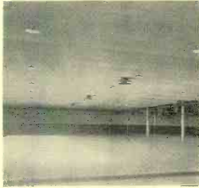
Fig. 25. Chandelier-type speakers with their 360-degree, slightly downward distribution pattern provide complete sound coverage of this roller skating floor of 100,000 sq. ft. with an acoustically deadened ceiling only 15 feet above the floor.
