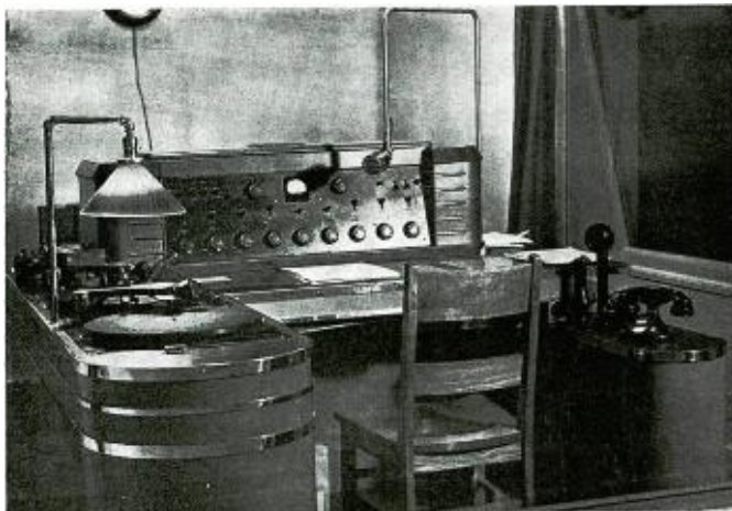
Typical 20 series console installation at CKTB, St. Catharines, Ont., Canada
