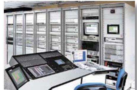
Route 5000/53 — Master Control Room of MediaCorp, Singapore
