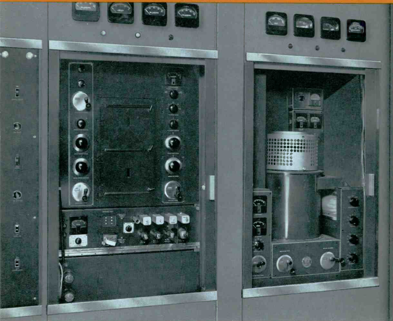
Visual transmitter section of the 10 kw driver used for the low power section of the TT-50AH transmitter. Photo shows visual driver chain and r-f amplifier cabinets.
