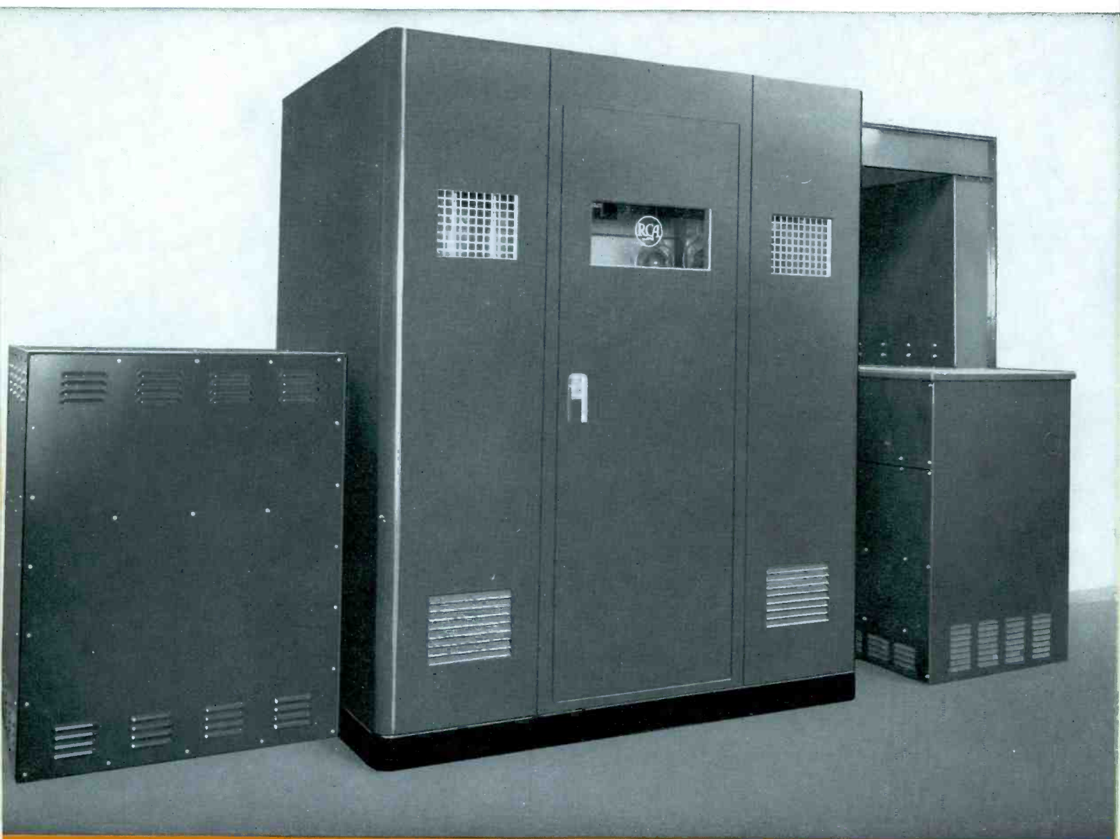
Photo of high voltage rectifier cabinet with high voltage plate transformer on right and filter reactors on the left. Ductwork is pictured at the right top of photo.
