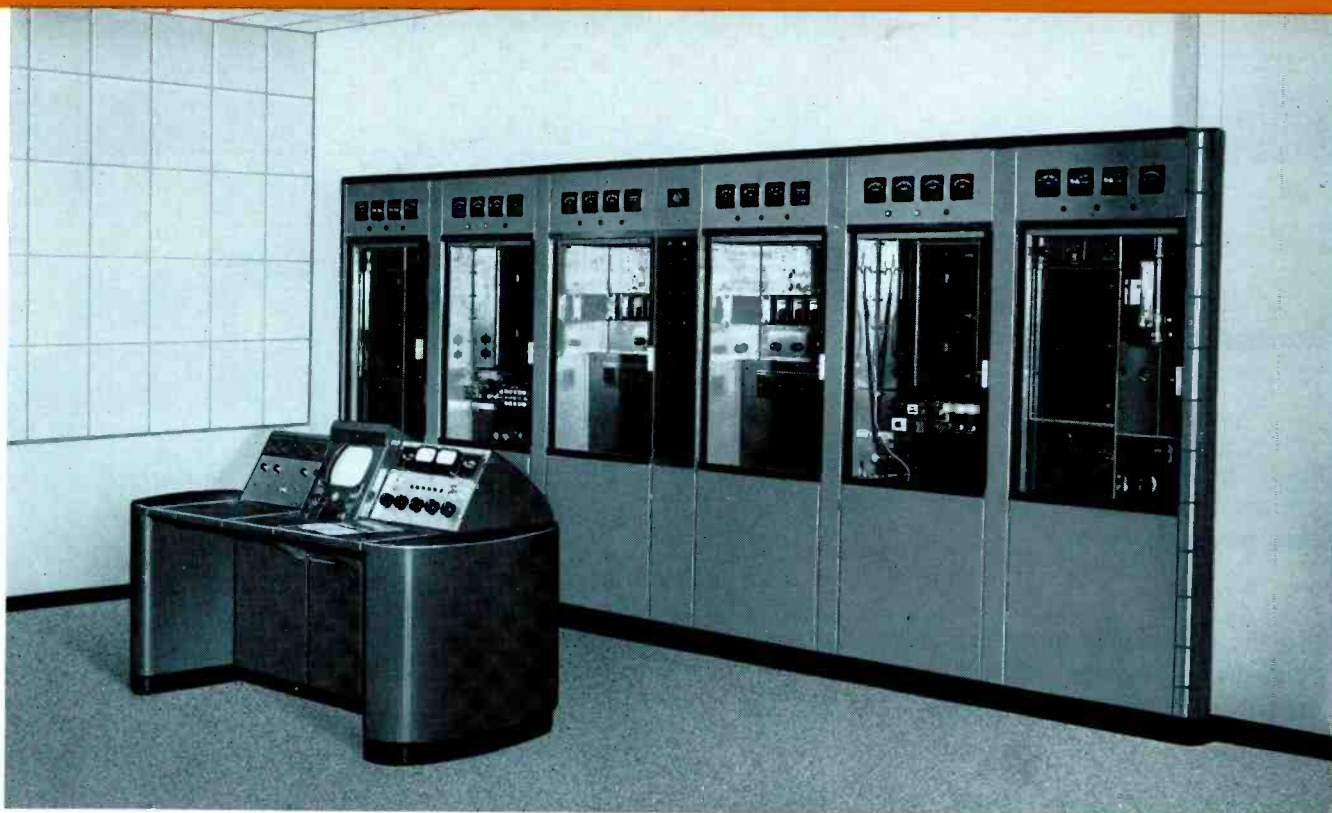
Typical transmitter installation showing the use of the TTC-1C Transmitter Control Console.
