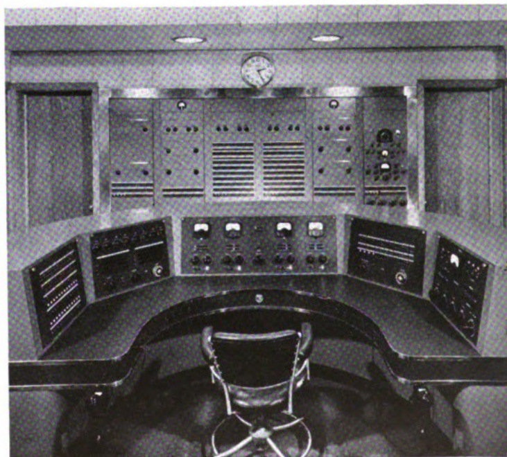
Master Control Room Speech Input of WLS.
