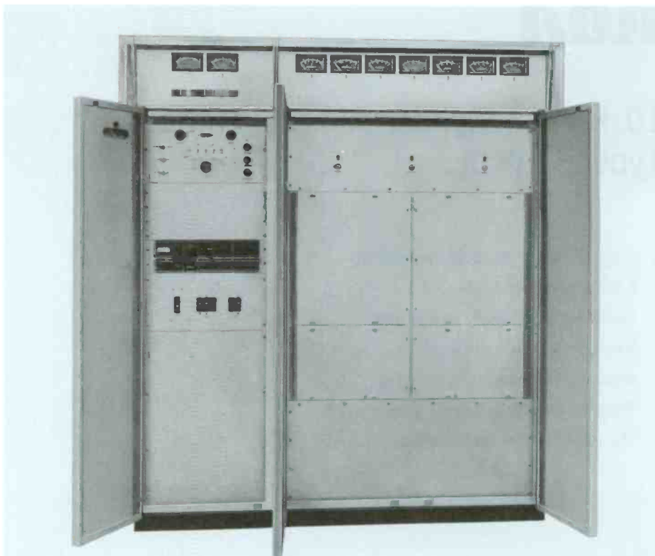
Front view, doors open. Note exciter unit.
