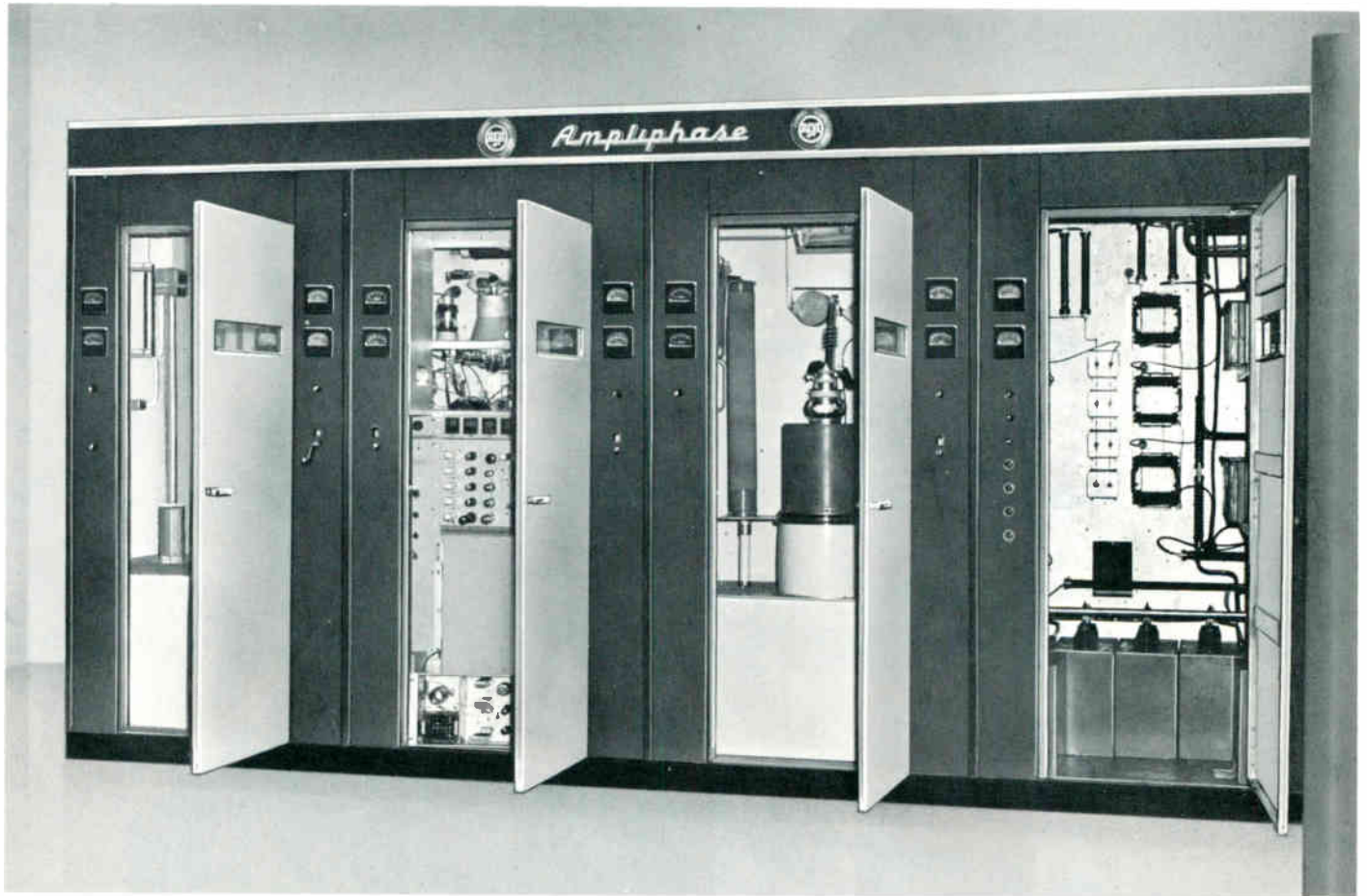
Compact in-line construction of BTA-50H1 showing left to right, left hand power amplifier, exciter, right hand power amplifier, and rectifier-control cubicle.
