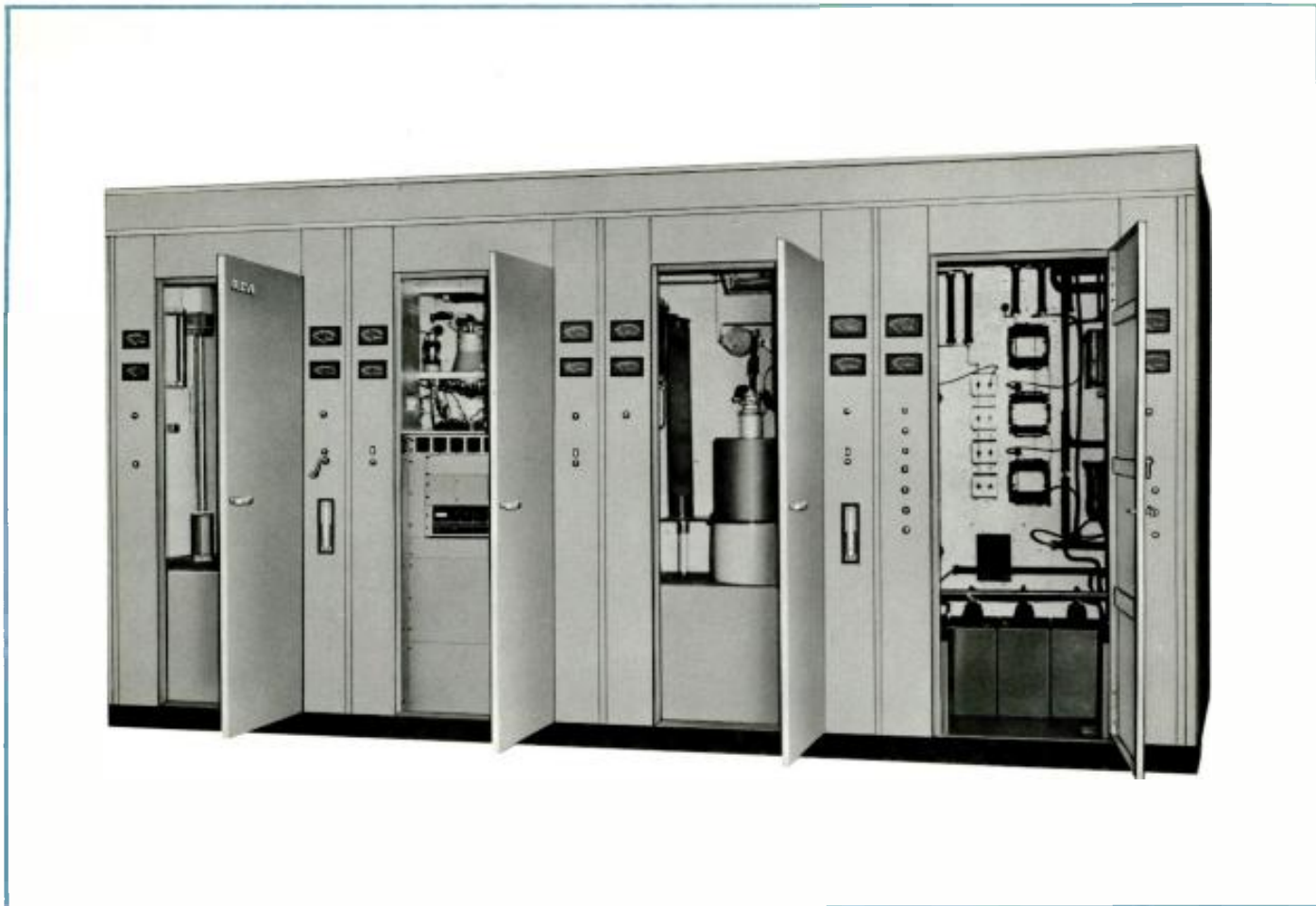
Compact in-line construction of BTA-50J showing left to right, left hand power amplifier, exciter, right hand power amplifier, and rectifier-control cubicle.
