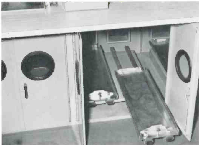
Shown is a typical video production desk with trays for field camera control units on the formica top and a forced air cooled compartment underside for field power supplies.
