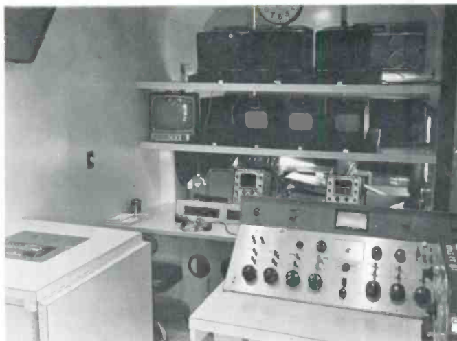
Typical interior of a TJ-70 series unit which has a video control desk in front, switcher and video desks in the middle and a TR-5 Tape Recorder at the rear. Shown is the view from the BC-8A Audio Console overlooking the three 14-inch production monitors, three 8-inch cameras, monitors and video control wedge with space for four CRO's in field cases.
