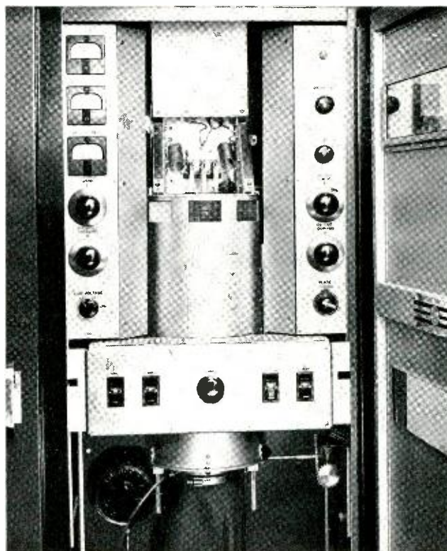
FIG. 3. Closeup view of the final stage of the 2 kw transmitter showing the RCA 5762 air-cooled triode.
